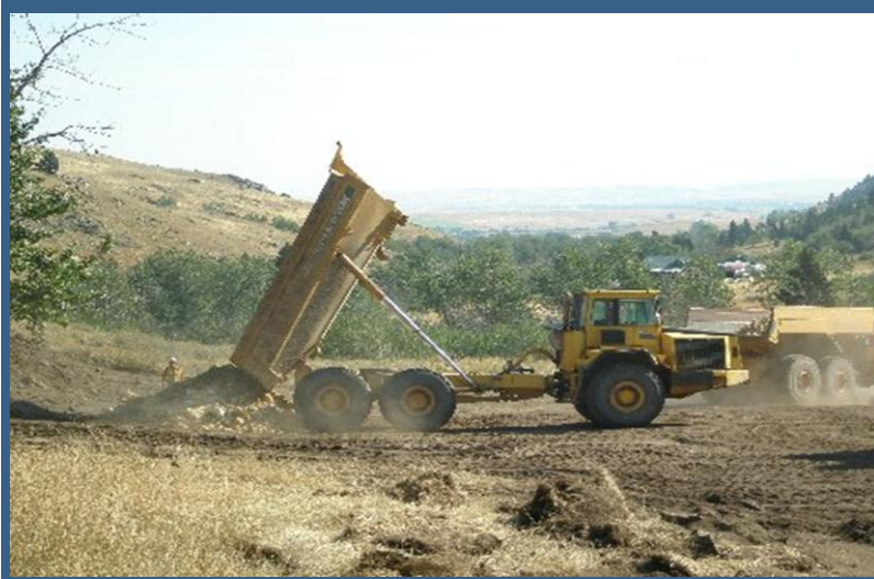
The first ore drop at the crusher site from the Mineral Hill Project!
